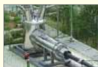
Terminal and connection box
