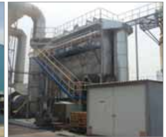
Dust collection facility in the melting furnace process
