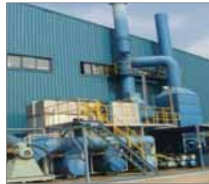
NOx removal facility(RTO+ SCR)
