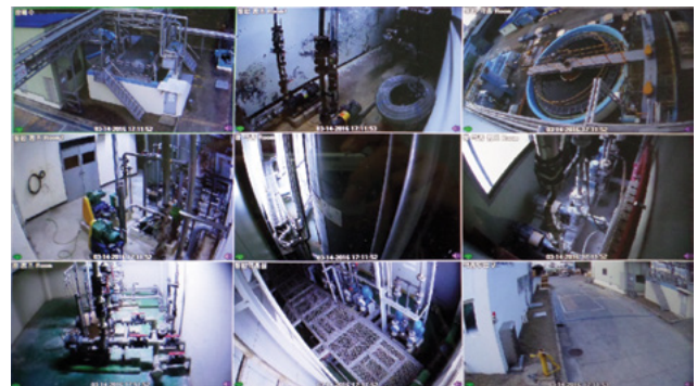
폐수처리장 Monitoring System
